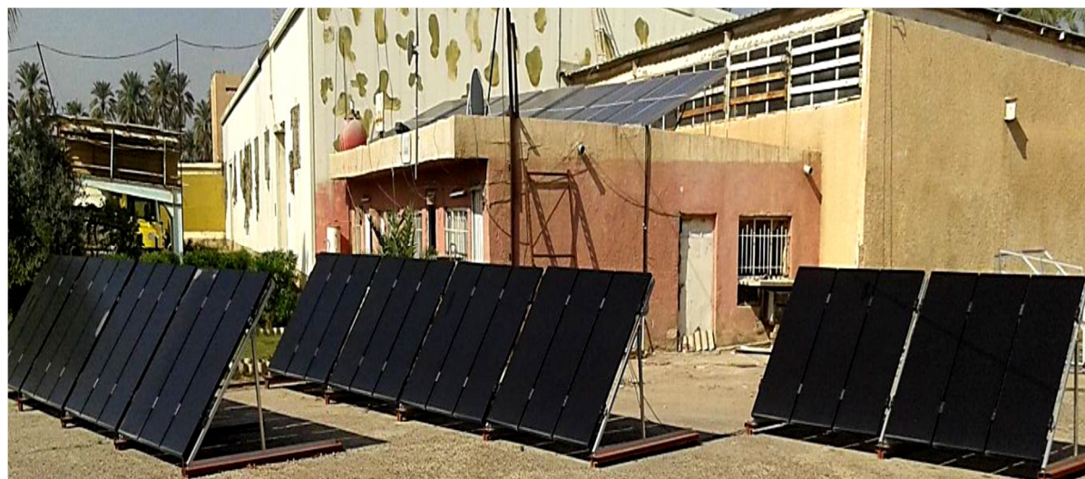
FIG. 1. Grid-tied CIGS PV solar system.
